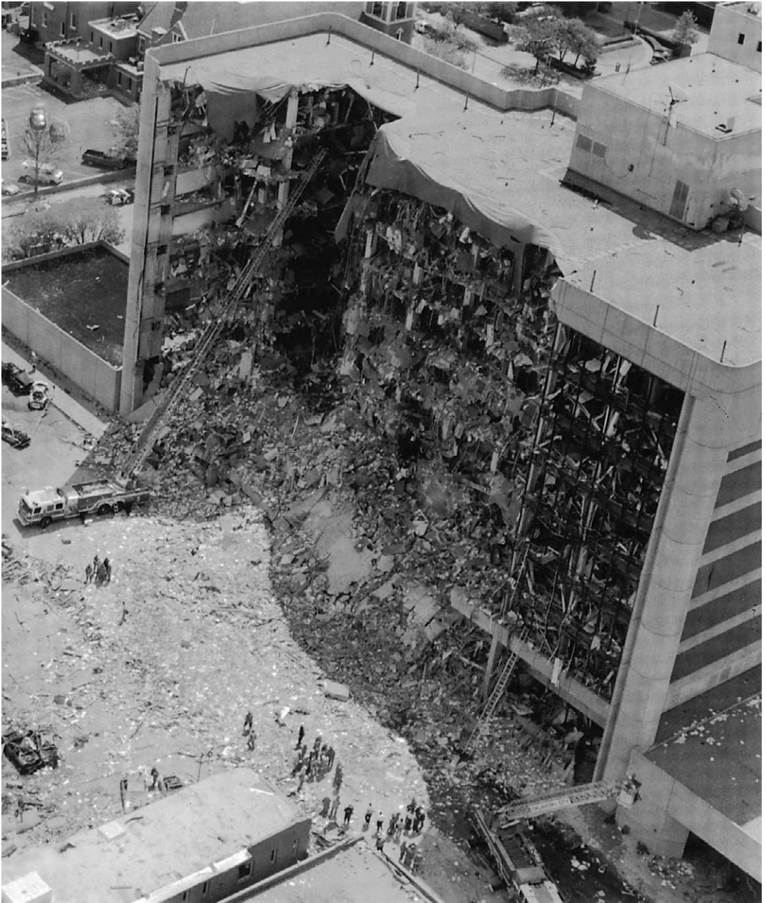
Figure 10.6 TERROR IN OKLAHOMA CITY. The Alfred P. Murrah Federal Building in downtown Oklahoma City sits in ruins after the April 19, 1995, devastating explosion that rocked the nation. Rescue workers using extension ladders work desperately to free survivors. Used with permission from AP/WIDE WORLD PHOTOS.
