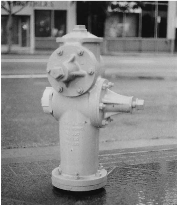
Figure 6.13 “California” wet barrel fire hydrant. Photograph by Roger Flores.
