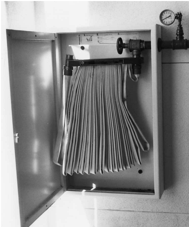
Figure 6.18 A fire hose cabinet. (This cabinet is located on the roof of a high-rise building in Los Angeles, where such installations are required by code.) Photograph by Roger Flores.
