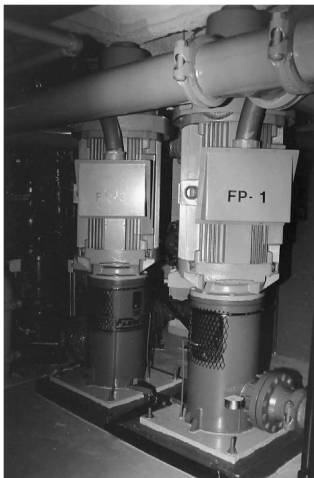
Figure 6.11 Two electric fire pumps located alongside each other in the fire pump room of a high-rise building. Photograph by Roger Flores.
