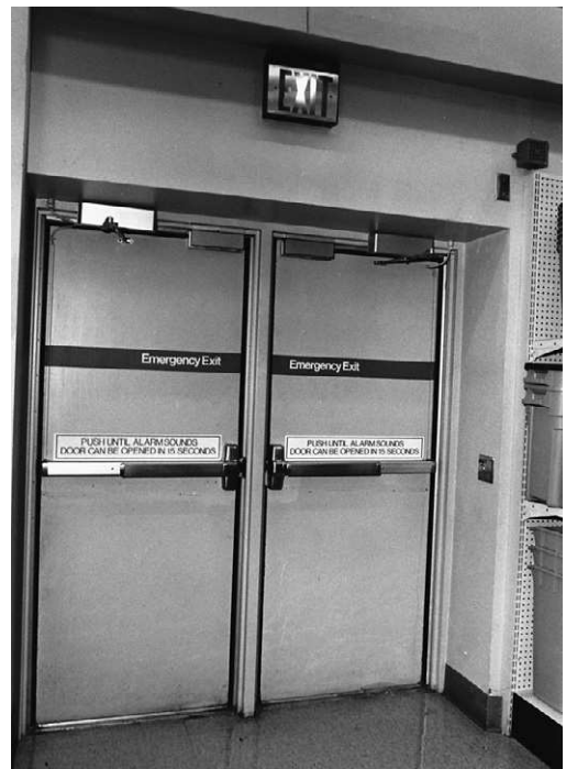
Figure 5.22 Pair of emergency exit fire doors equipped with a delayed exit system. Note the rim-mounted push bar, the surface-mounted electromagnetic lock at the top of each door (close to the center divider), and the key switch that operates the electromagnetic lock immediately adjacent to the pair of doors on the right-hand side. (Each door is also equipped with surface-mounted automatic door-closing mechanisms.) Courtesy of Von Duprin, Incorporated, Indianapolis, IN.
