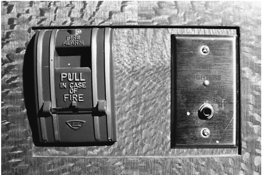
Figure 6.3 Example of a manual fire alarm station on the left-hand side and a fire department voice communication system jack on the right-hand side. Photograph by Roger Flores.
