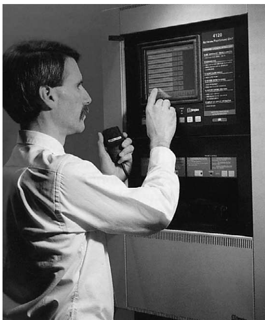
Figure 6.2 A Building Fire Safety Director identifies the type of fire detection device in alarm and its location before making a public address announcement to the occupants of a modern high-rise building. Courtesy of SimplexGrinnell, A Tyco Company.
