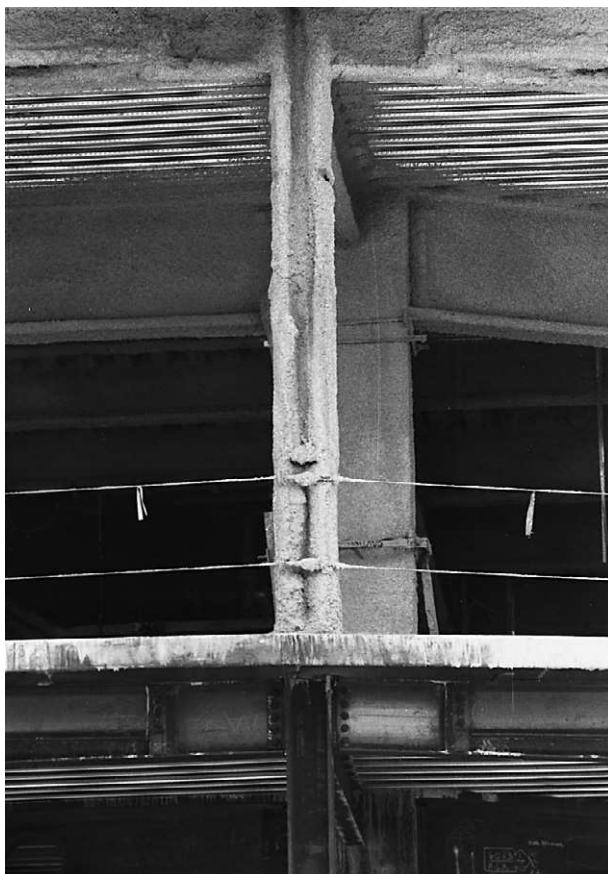
Figure 3.2 Floors of a steel-frame high-rise building exposed during construction. Note the corrugated-steel decks and sprayed-on fireproofing insulation. Photograph by Stephen Lo.
