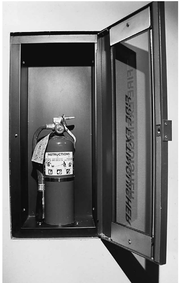
Figure 6.23 Portable stored pressure ABC multi-purpose extinguisher housed in a cabinet. Photograph by Roger Flores.
