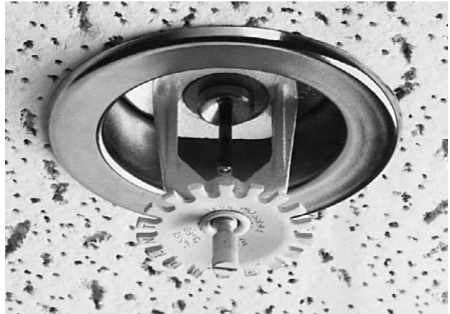
Figure 6.15 A recessed sprinkler protruding through the ceiling. Courtesy of Viking Corporation, Hastings, MI.
