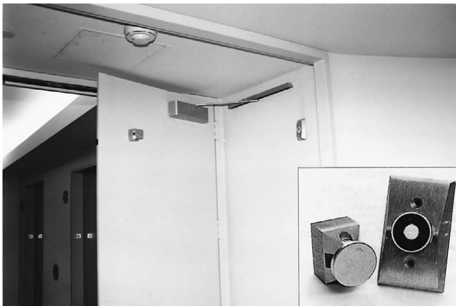
Figure 5.27 Elevator lobby doors closing on activation of the building's fire life safety system. Insert , a close-up of an electromagnetic door holder, courtesy of Sentrol, Inc., Portland, OR.
