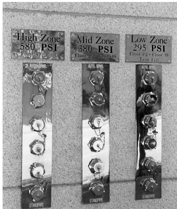
Figure 6.12 Fire department connections serving high, mid, and low zones of a modern high-rise building. Photograph by Roger Flores.
