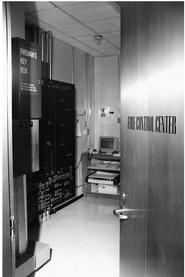
Figure 6.1 Example of a Fire Control Center. Photograph by Roger Flores.
