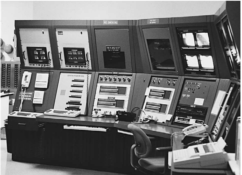
Figure 5.2 An enclosed Security Command Center. Photograph by Roger Flores.
