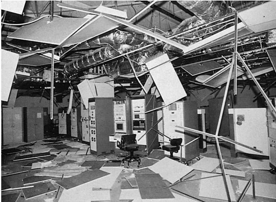
Figure 10.17 During the 1994 Northridge earthquake these tall, castor-mounted computer cabinets rolled across the floor of a second-story room without overturning. Unfortunately, the newly installed ceiling and lighting fixtures did not fare as well. Courtesy of Dames and Moore/URS Corporation, A Special Report on the January 17, 1994, Northridge Earthquake .
